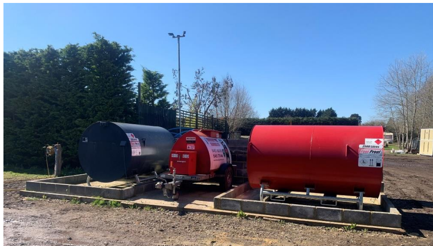
Fuel Bunding on Officers Site Visit dated 4 April 2023
